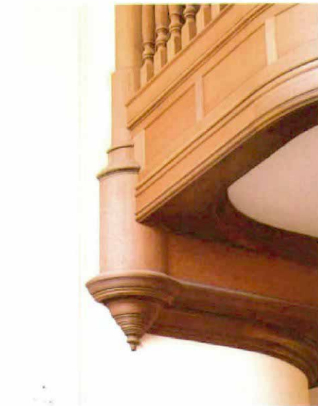
Formal crown molding was designed to split into two separate crowns where it makes its turn into the lobby. At top, the radiused crown awaits a butt-joined section of straight crown to tie it into the turned drum. Note the blocks screwed to the wall to secure the crown. The finished installation (above) shows how the various trim elements come together, a major exercise in scribe-fitting where the crowns meet the drum.
